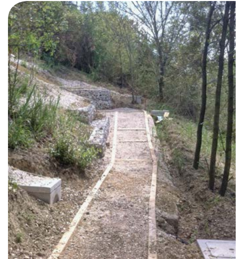
System of infiltration trenches, urban trekking path Monte Mario, Rome, Italy, 2016. (Simone Amantia Scuderi, Rome, Italy – photo Simone Amantia Scuderi).
