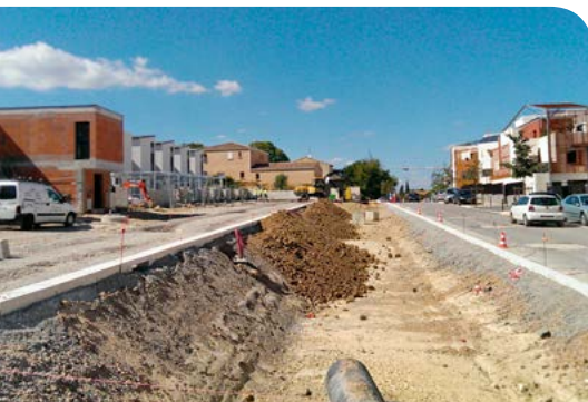
Infiltration swale, under construction, Roque Fraïsse Ecodistrict, Montpellier, France, 2016. (Les Ateliers UP+, Christian Matteau Landscape Architect, Montpellier).
