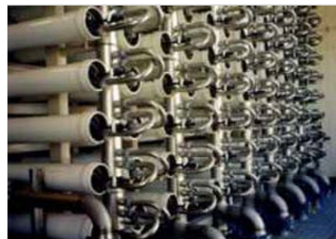
At West Basin Wastewater Treatment Plant in California, reverse osmosis, an advanced treatment process, is used to physically and electrostatically remove impurities from the wastewater.
